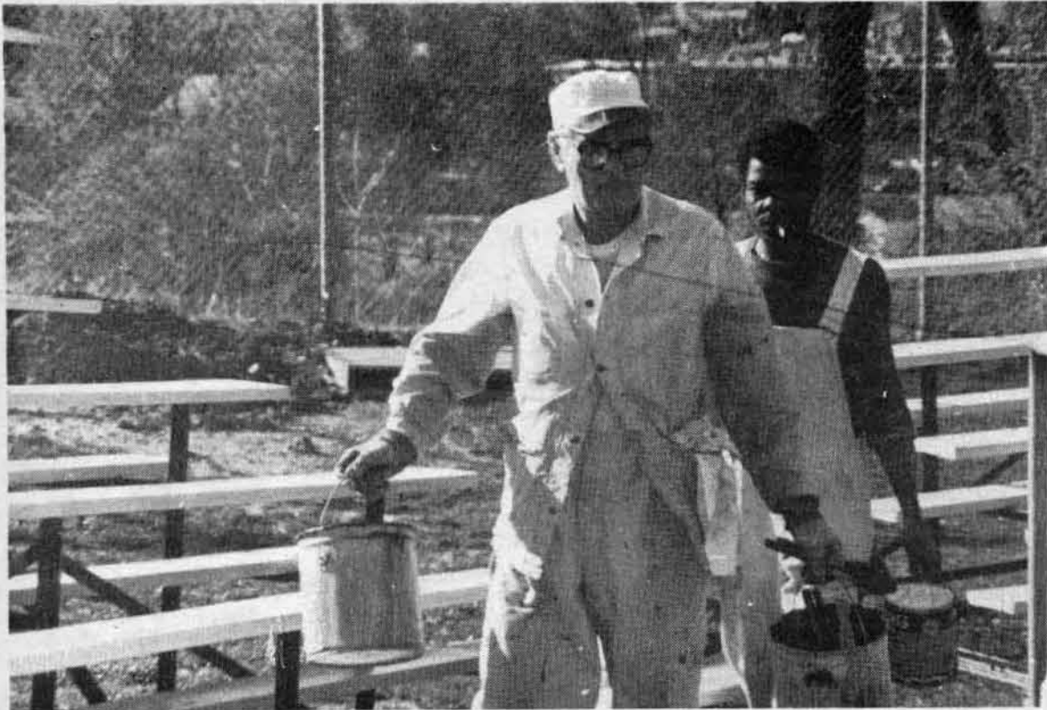
PUTTING N A NEW COAT: Two Physical Plant workers take advantage of the spring weather to repaint the bleacher located north of the Multi-Purpose Building. [Photo by Scott Petersen].
